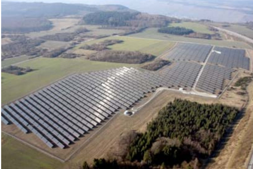
Figure 4. Mehringer Höhe Solar Park I, Germany - www.juwi.com
